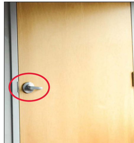
Even door handles can provide an attachment point for a ligature.
